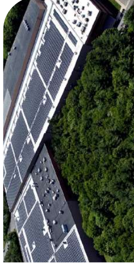
Performance Line Solar Panels Rooftop Installations
