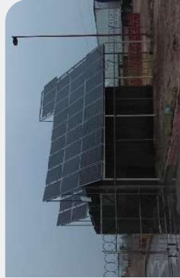
Solar panels installed atop our organic garden
